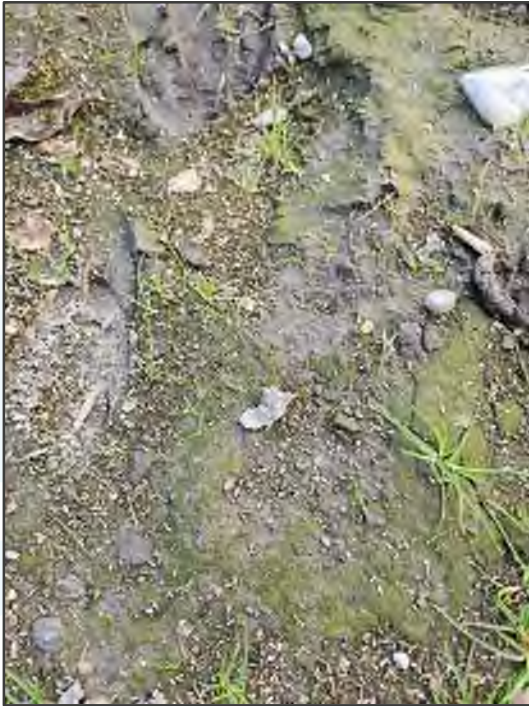
PHOTO NO. 136: Wetland Y - Algae and Cracks
