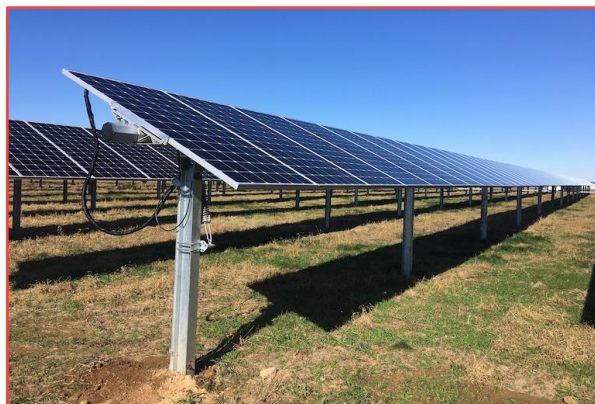
Figure 1: Example of Single-axis Tracking System, Ground-mounted Solar PV Arrays
