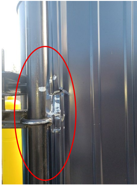
Damage impeding function
