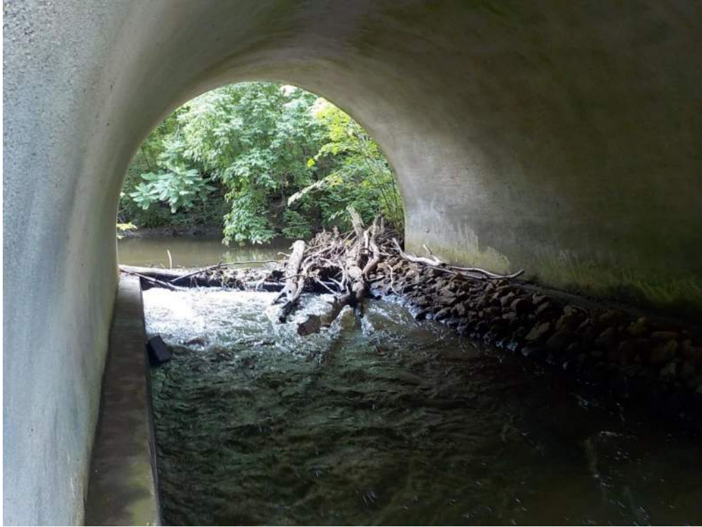
Debris in stream
