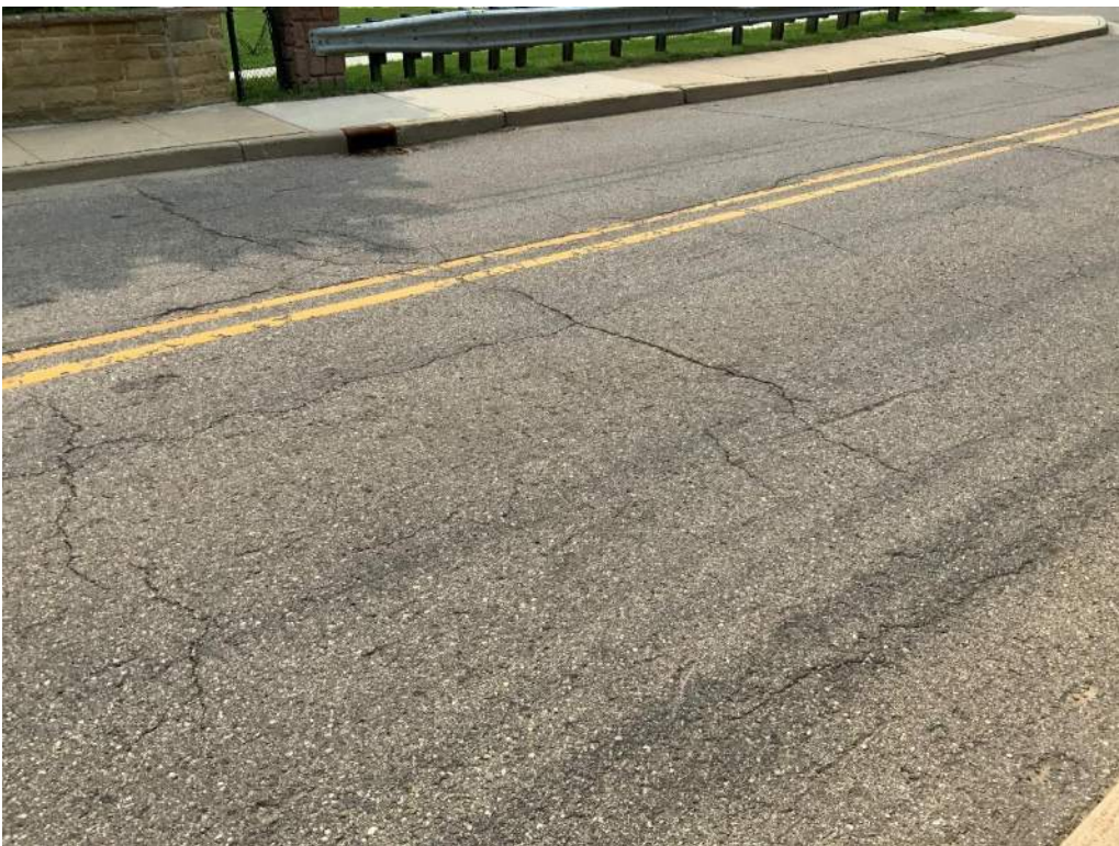
Cracks in wearing surface
